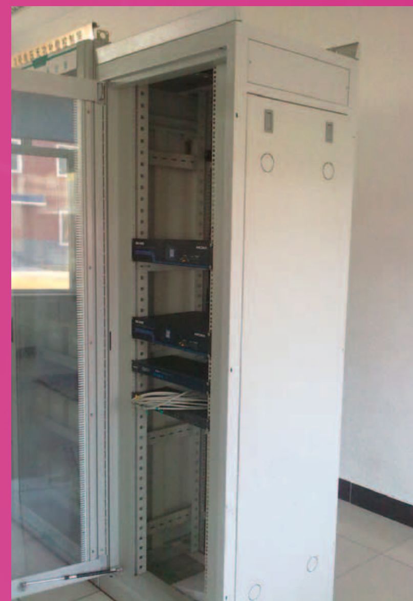
Wind Farm Voltage Controller
