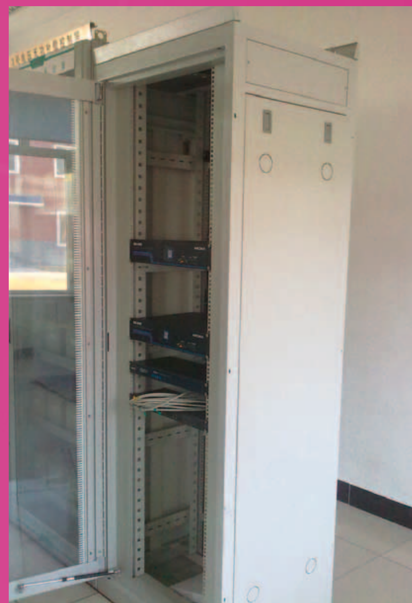
Wind Farm Voltage Controller
